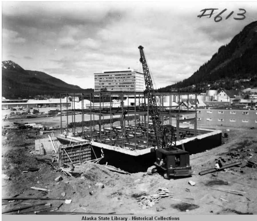
Figure 2. Photo showing the basement wall and the steel framing system of the building. The background also shows the 8-story Federal Building.
