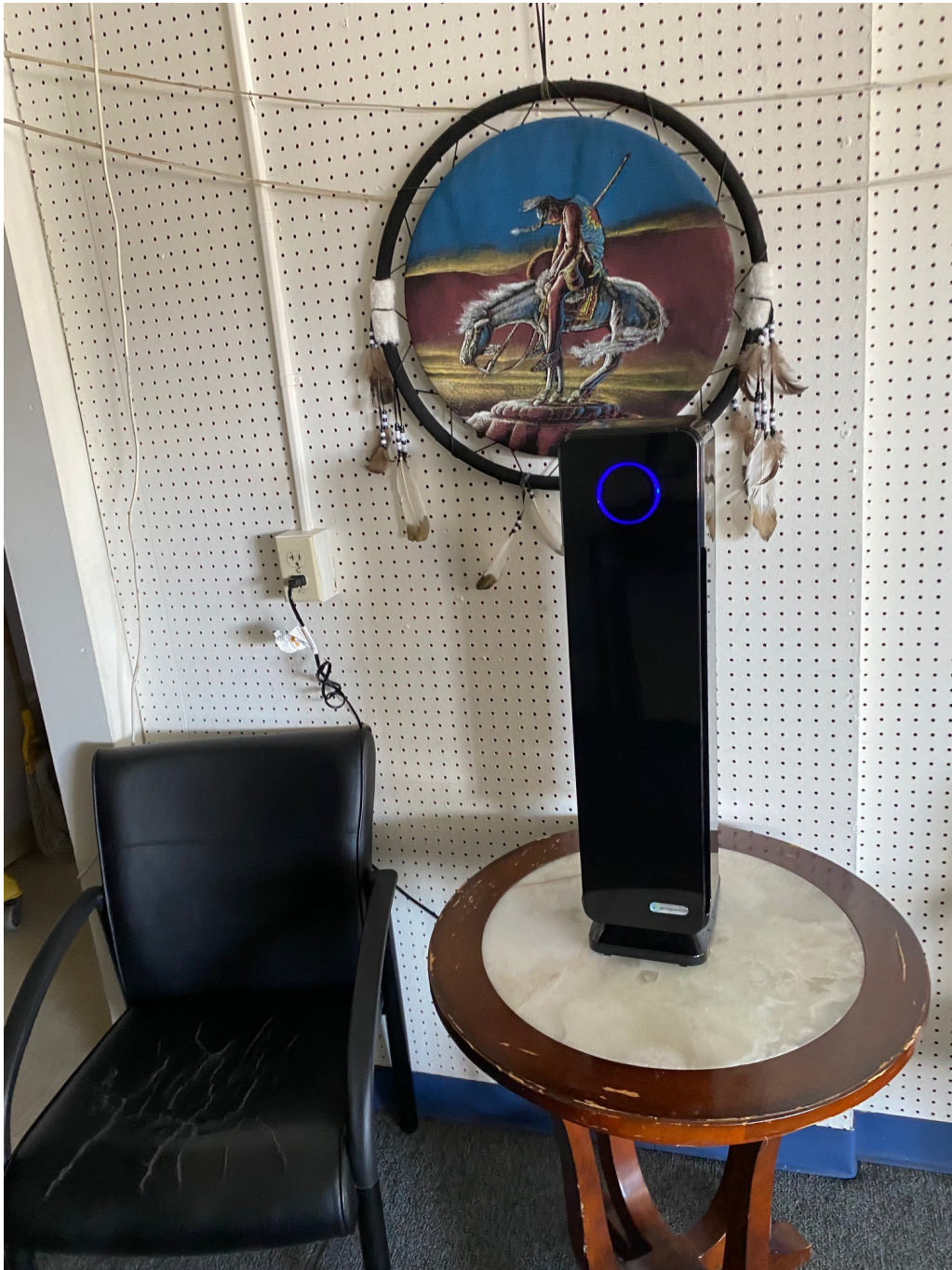
One of twelve UV & HEPA Air Cleaners
