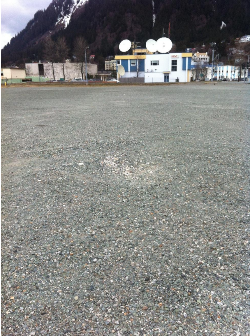
Photograph 9. Deeper pothole located in the southern portion of the property mid-site.
