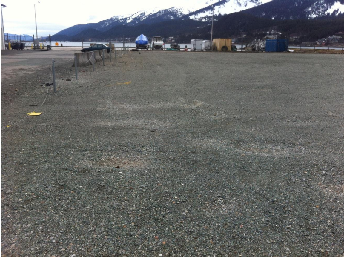
Photograph 7. Series of potholes located near the entrance/exit of the Whittier Street vehicle access.
